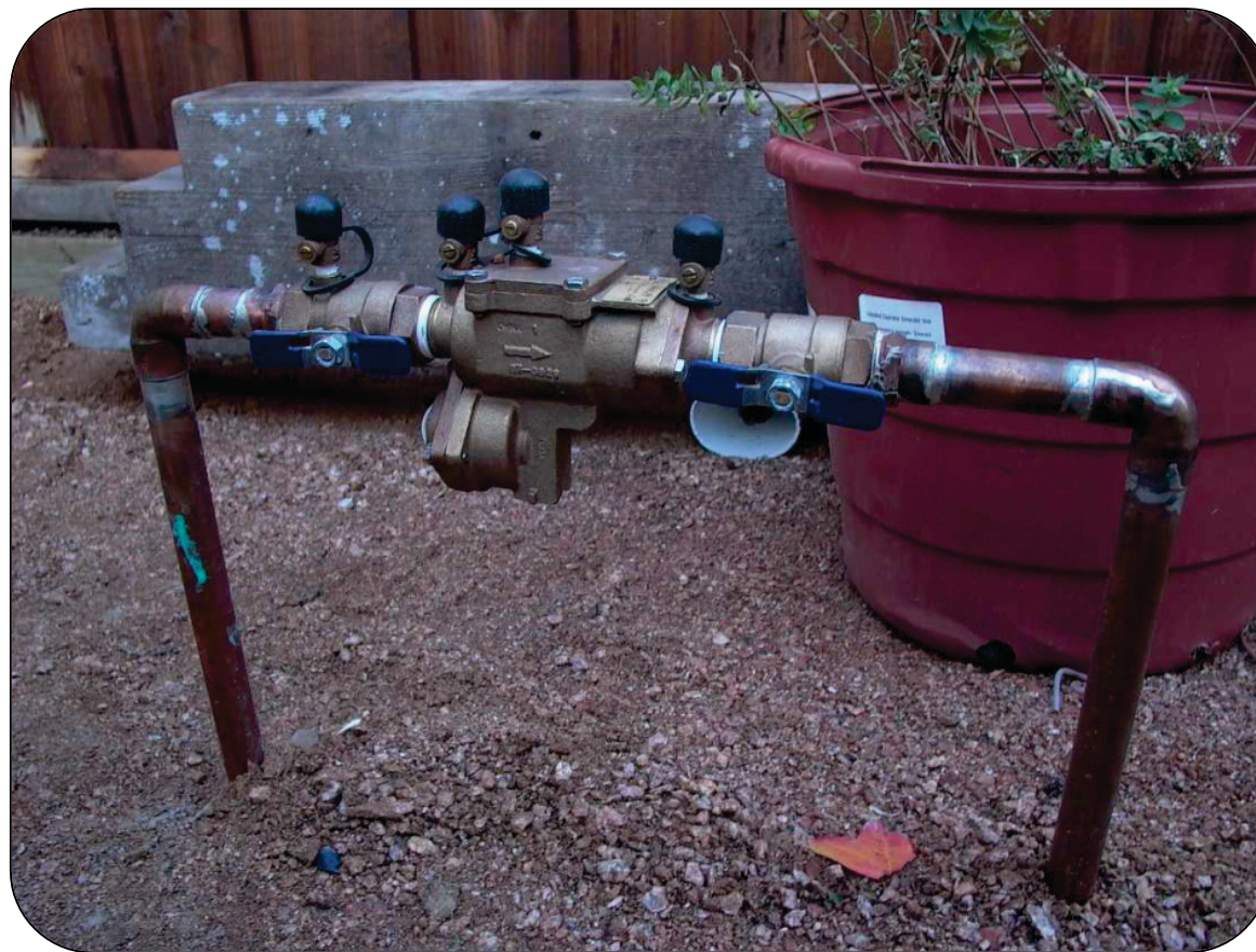
Backflow prevention device, McMahan residence, Dallas, Texas.
