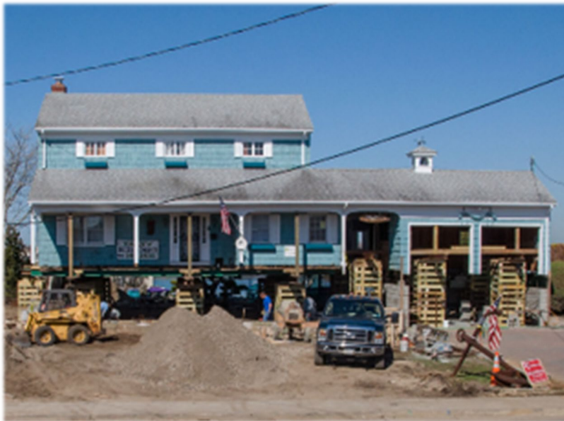
Figure 1. Photo shows a house elevated on temporary supports while crews work on a new foundation.
