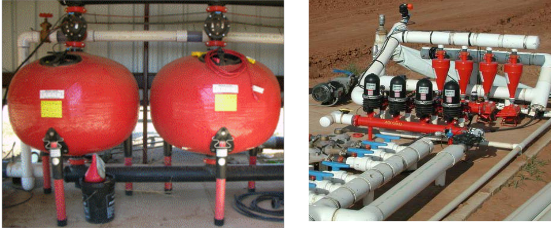
Figure 2.21. Sand media filters (left); hydrocyclone and disk filters (right) remove particulate matter from water to reduce risk of tape or emitter plugging.
