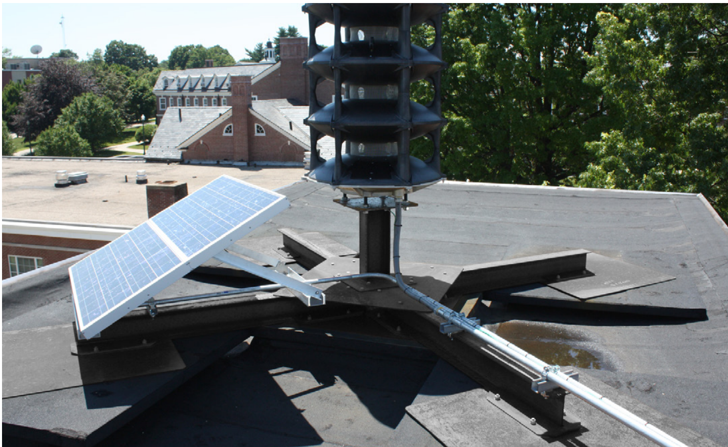
Whelan WPS-2903 siren mounted on a roof
