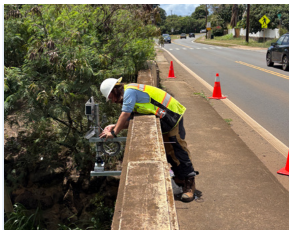
Installation of river gauge on a roadway
