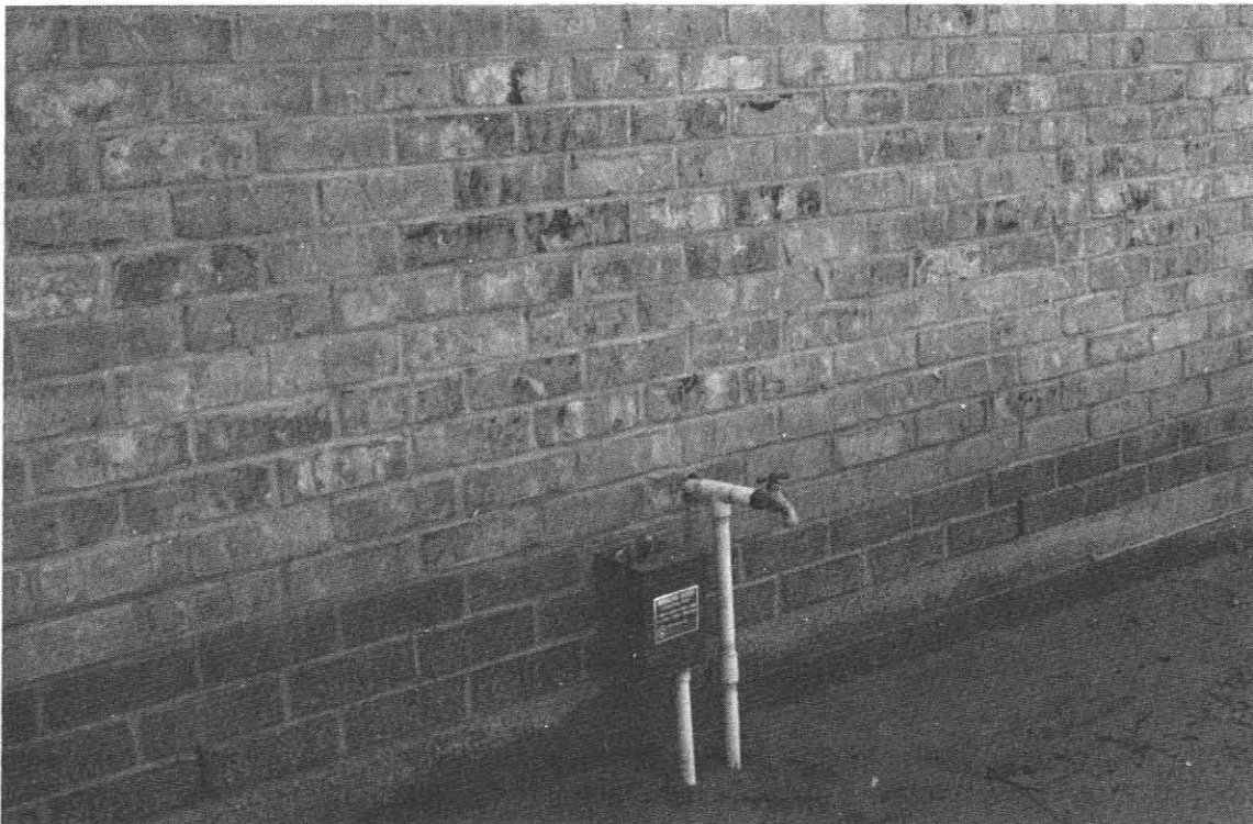
Figure 9-7.—Wellhead of Heat-Pump System Injection Well, Montgomery County
