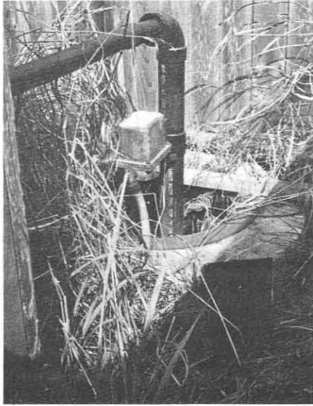
Wastewater holding tank, submersible pump, and transmission line.
