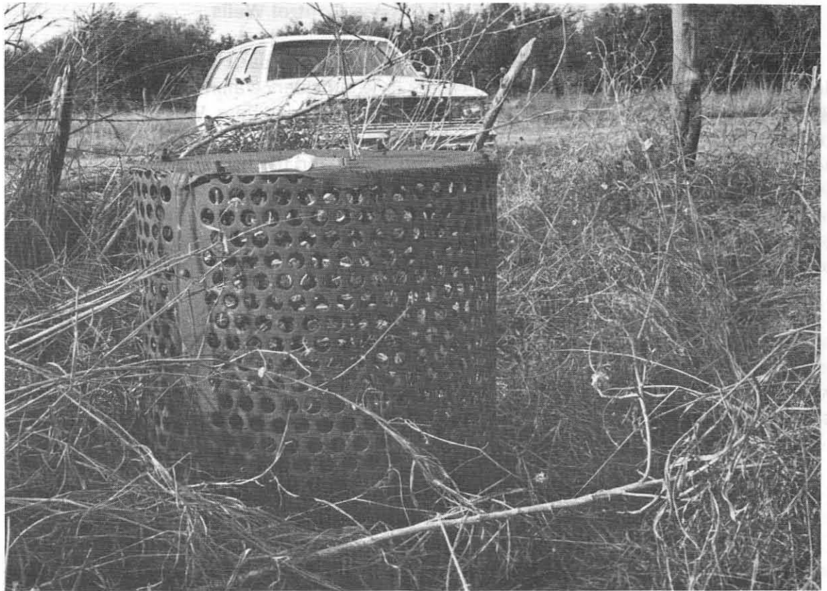
Figure 8-16.—Recharge Drain Well in Rocksprings, Edwards County
