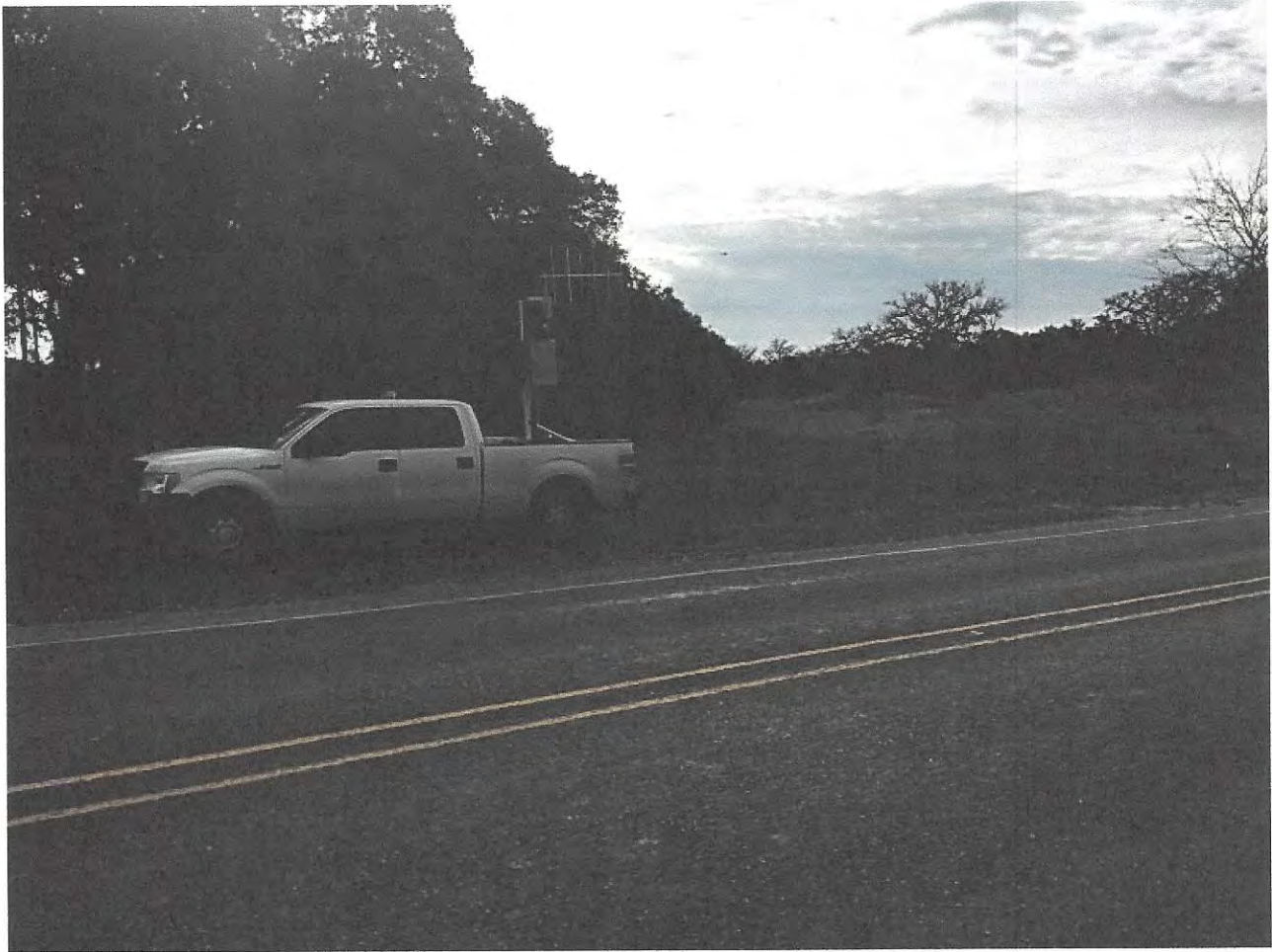
SABINAL RIVER AT RANCH ROAD 187 29.6664180, -99.5443840 RAINFALL GUAGE AND STREAMFLOW MONITORING EQUIPMENT
