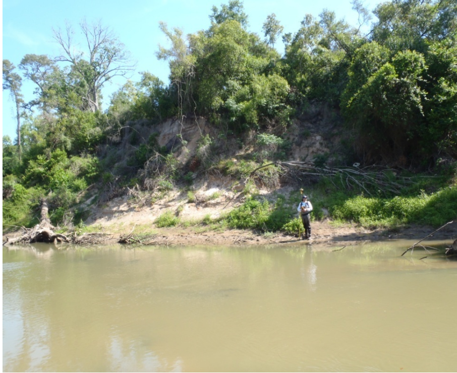
Figure B9: Bank Erosion/Failure on Buffalo Bayou at Memorial Park
