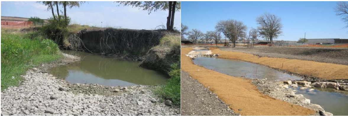
Figure 13: Typical Erosion at East Salitrillo Creek Prior to Construction (left) and View of Project During Construction (right).
