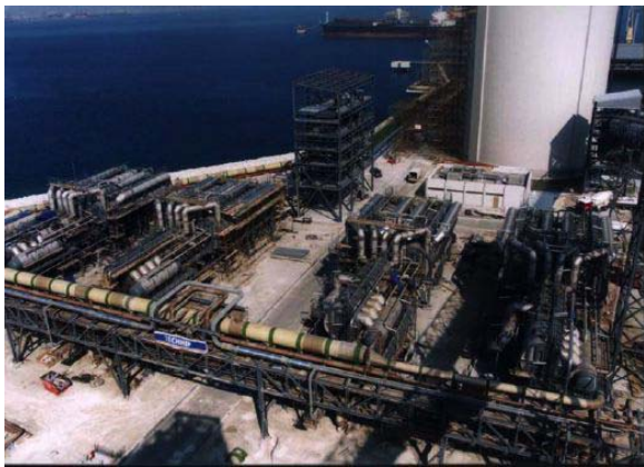
Figure 6 Coke calcining facility for aluminum smelter
