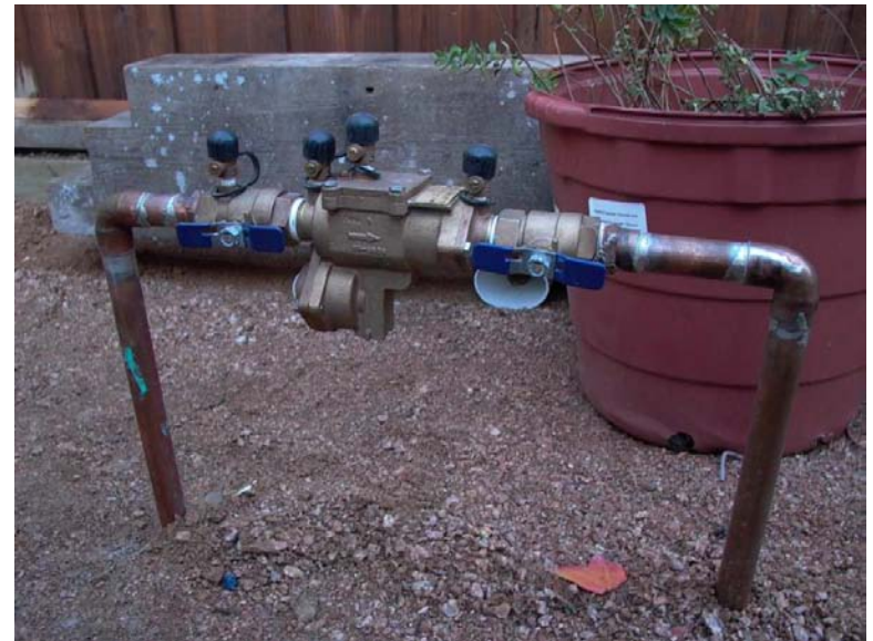
Backflow prevention device, McMahan residence, Dallas
