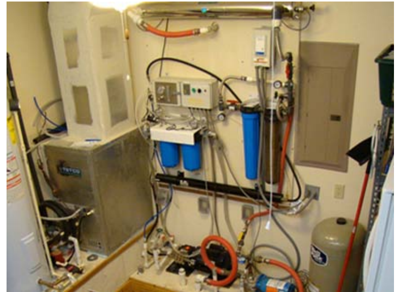
Sediment and sand filters, UV lamp, and pumps, Moore residence, Taft
