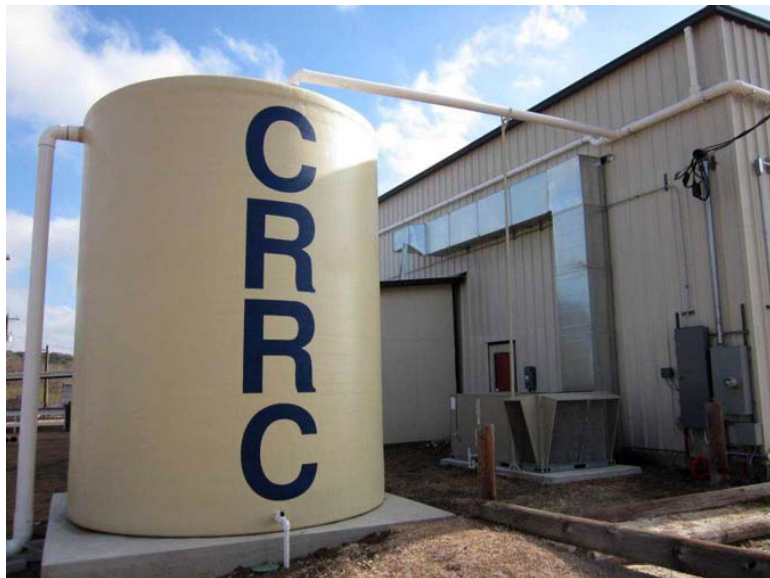
Fiberglass tank, CRRC, Canyon Lake
