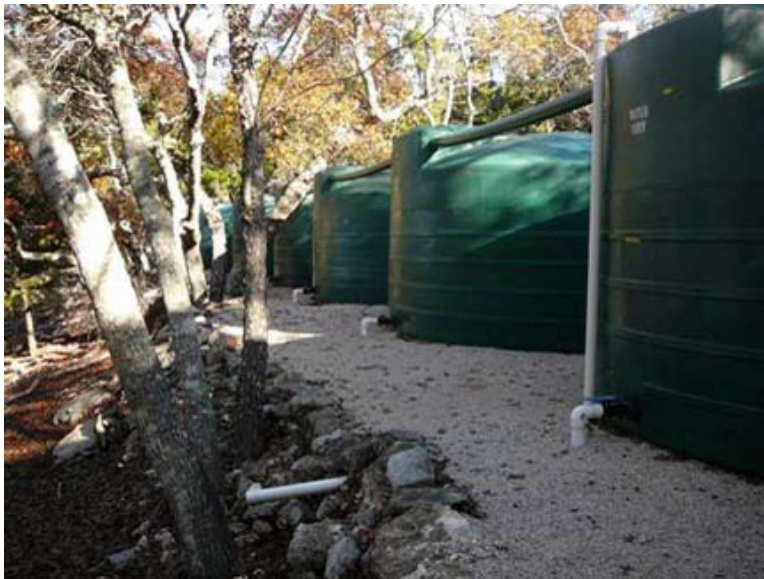
Polyethylene tanks (Kight residence, Boerne)
