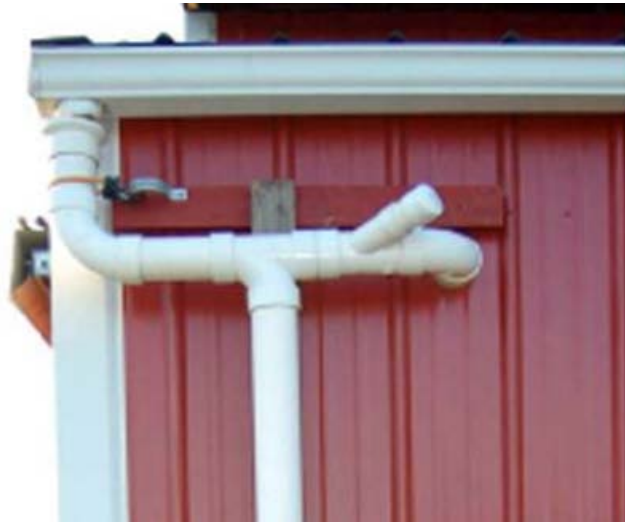
Roof gutter, Y valve connector and downspout on barn, Larrison residence, Georgetown
