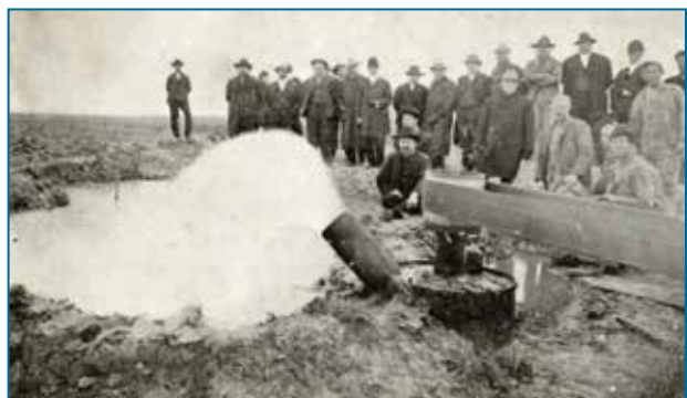
FIGURE 51. Testing a water well for rice farming near El Campo, Texas (circa 1910).
