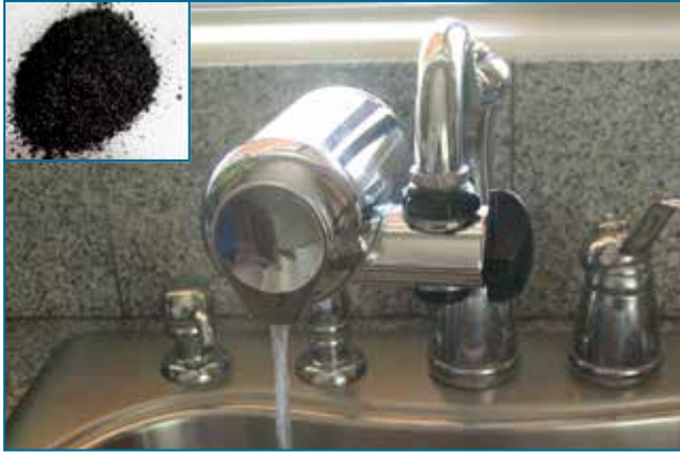
FIGURE 54. An activated carbon point-of-use treatment installed on a faucet; the carbon media is shown in the photo insert.
