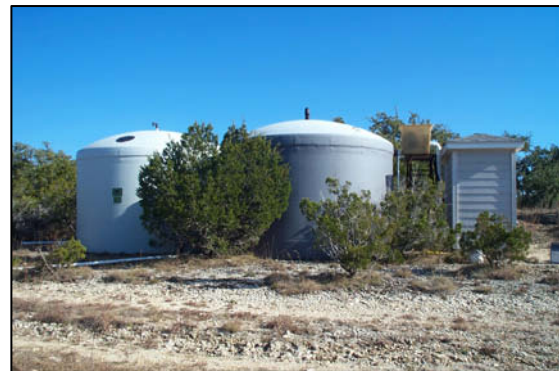
Figure 2-5. Two 10,000-gallon fiberglass tanks
