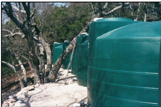
Figure 2-6. Low-profile 5,000-gallon polypropylene tanks
