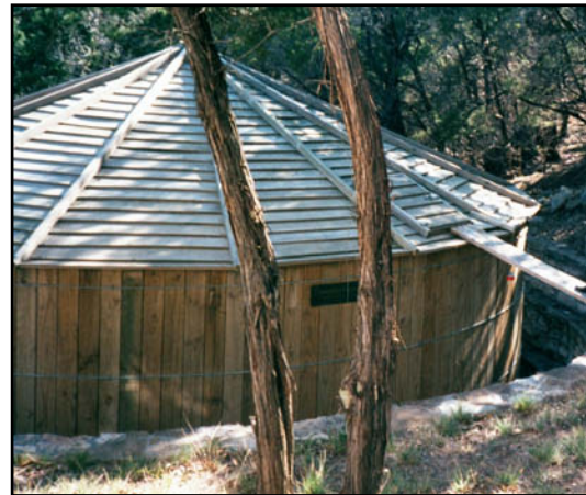
Figure 2-7. Installation of a 25,000-gallon Timbertank in Central Texas showing the aesthetic appeal of these wooden tanks
