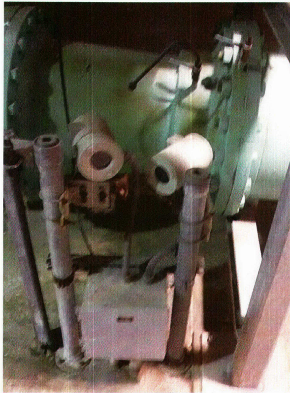
Figure 2.4: Venturi Flow Meter at Filter No. 7, instrumentation not connected (typical)
