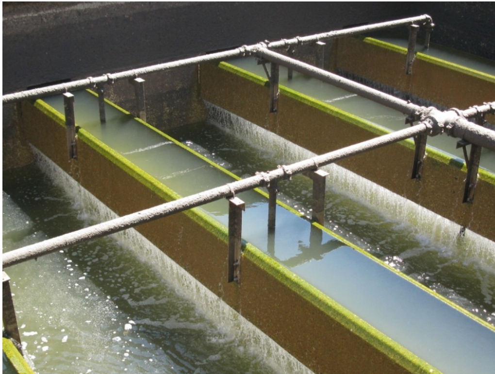
Figure TM2-1 – Filter in Filter Building 1
