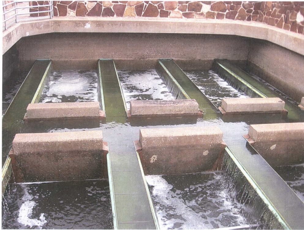
Figure TM2-2- Filter in Filter Building 2
