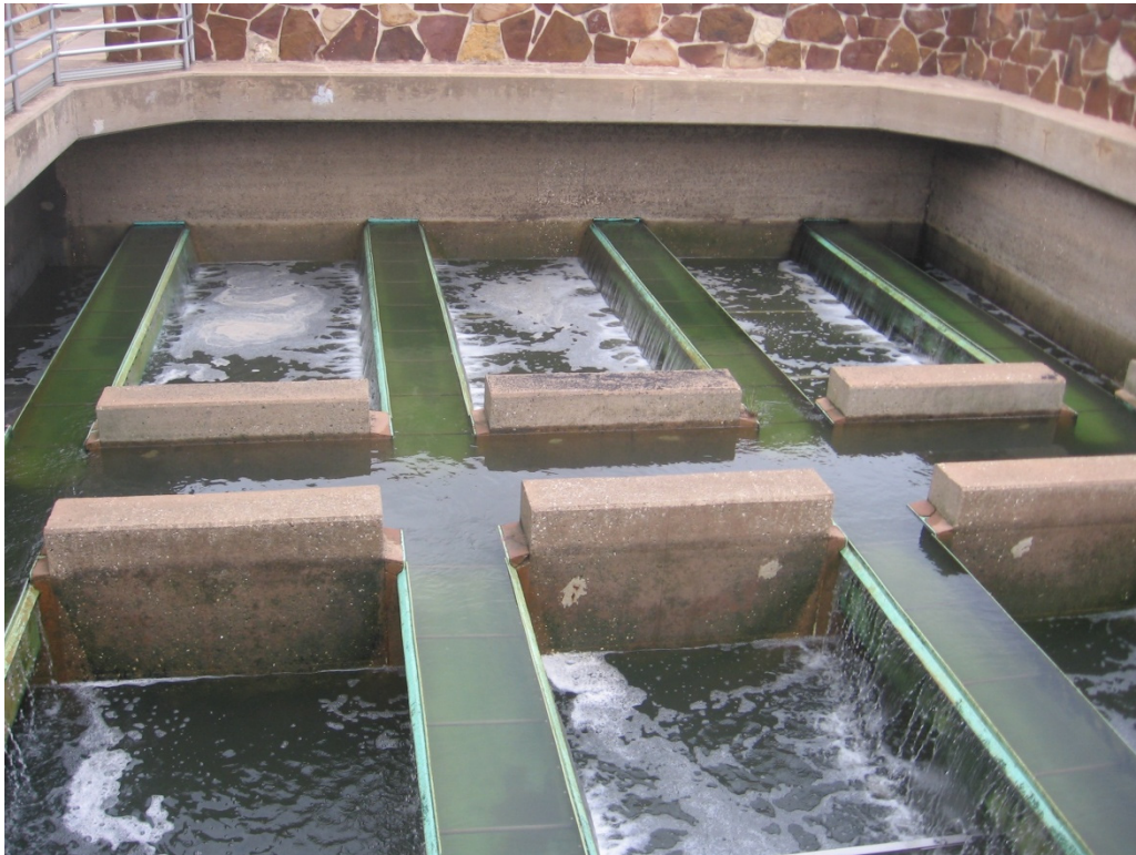
Figure TM2-2- Filter in Filter Building 2
