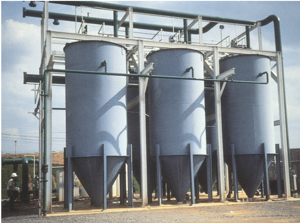
Figure TM2-12 - Upflow Filtration System
