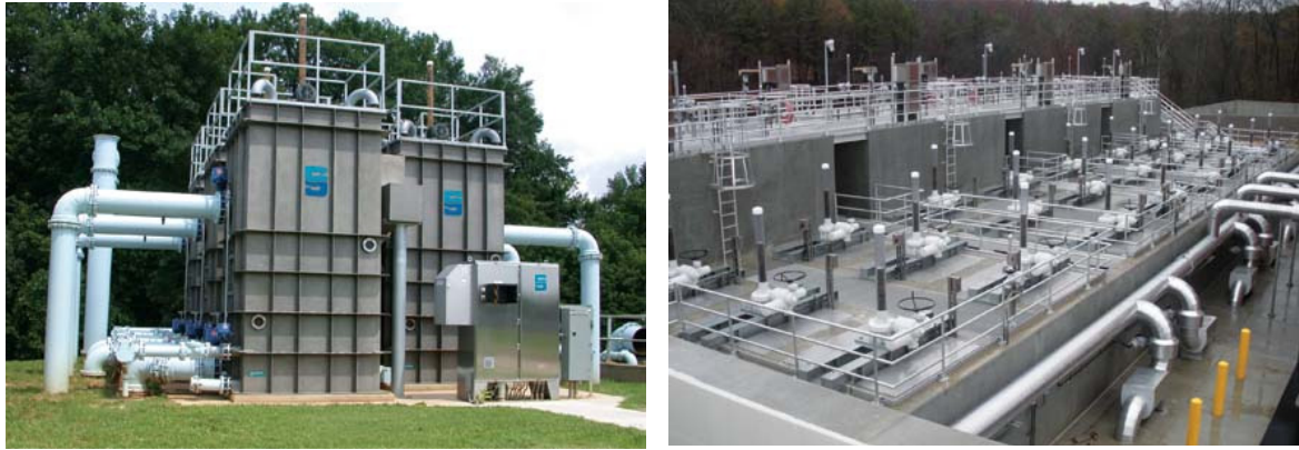
Figure TM2-14 – CMF Installations
