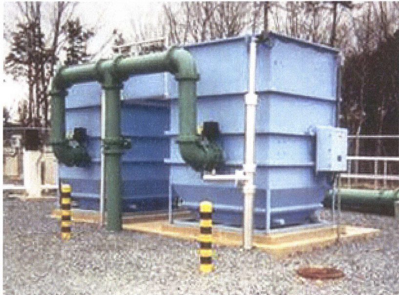
Figure TM2-16 - Cloth Media Filter Installation
