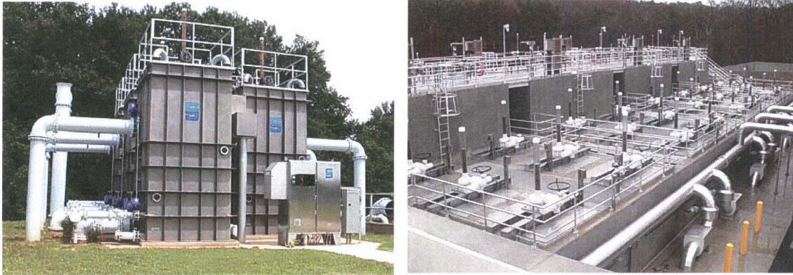
Figure TM2-14 – CMF Installations
