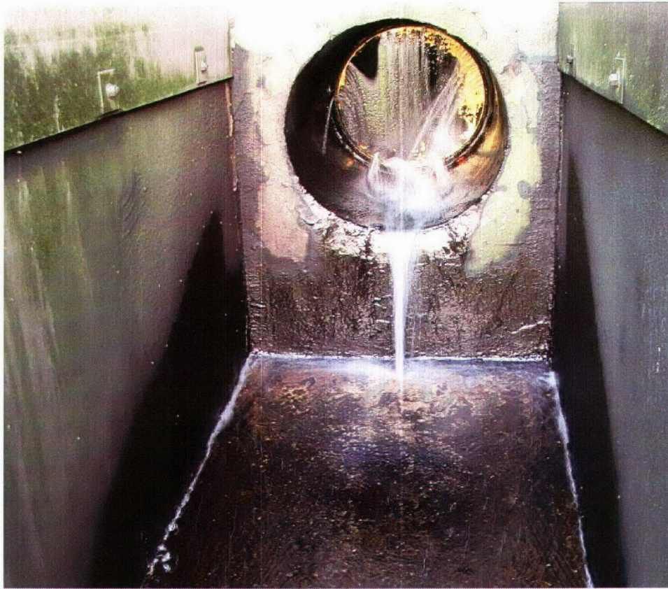
Figure 2.2 - Filter No. 12 Influent valve seat leaking. This condition is noted as typical during all observed backwash cycles
