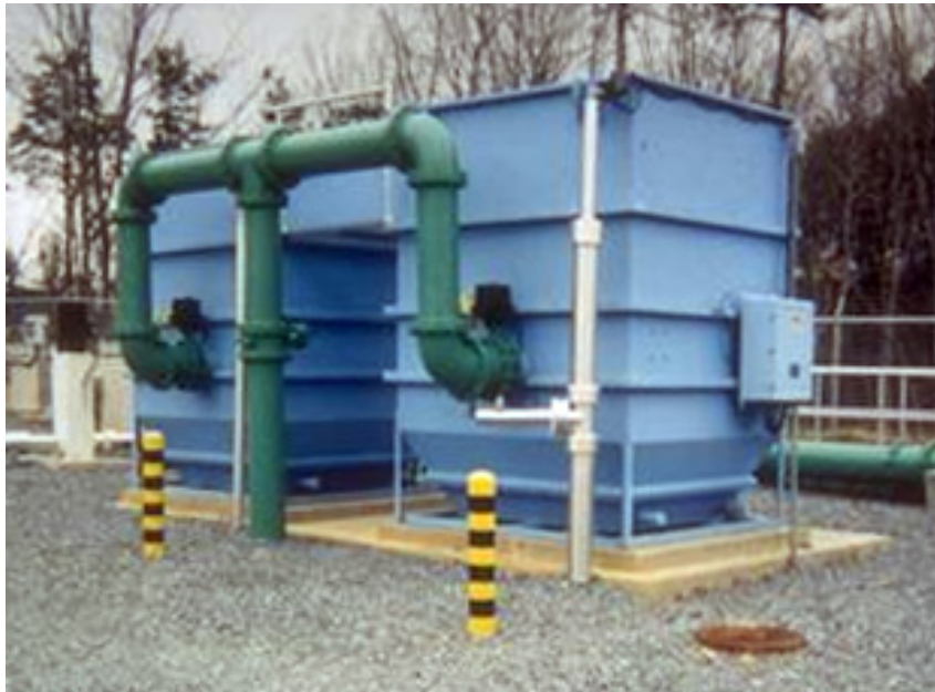
Figure TM2-16 - Cloth Media Filter Installation
