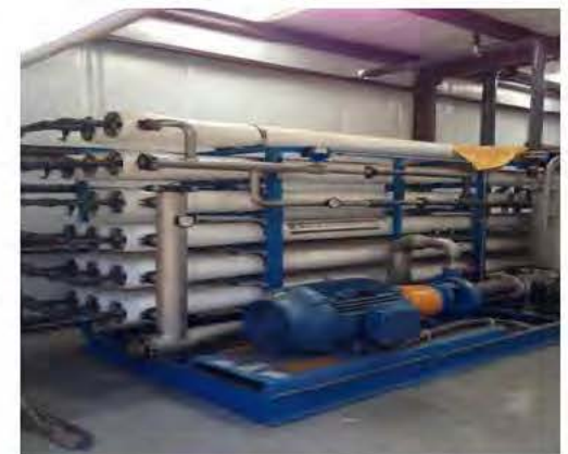
Ranchland Hills Country Club Hybrid Reverse Osmosis System 700,000 gallons/day or 16,666 barrels/day
