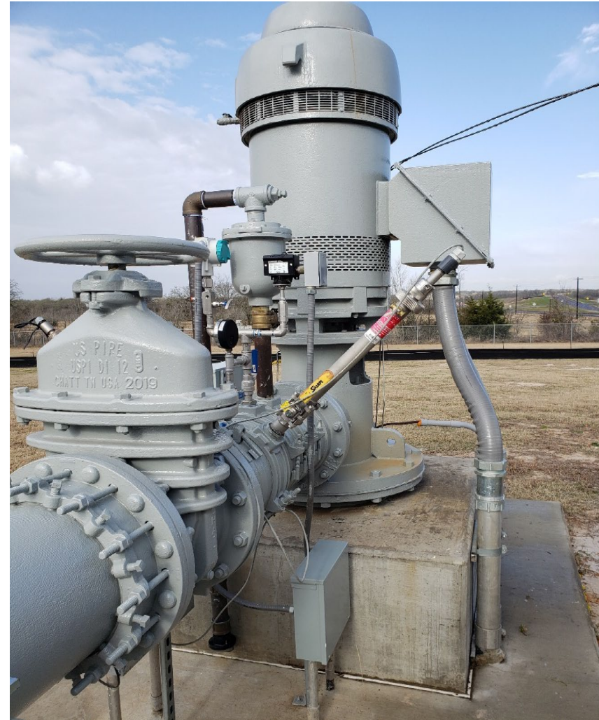
Aquifer Recovery and Storage Well – Well No. 10
