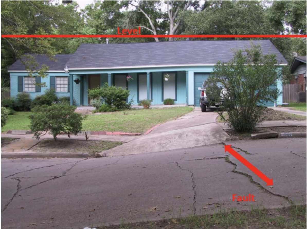
FIGURE 4-23. EXAMPLE OF FAULT IMPACTS ON A HOME IN GMA 14 (HOUSTON GEOLOGICAL SOCIETY, 2019)
