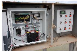
Close-ups from top left: HID auto-gates at work; actuator; control box.
