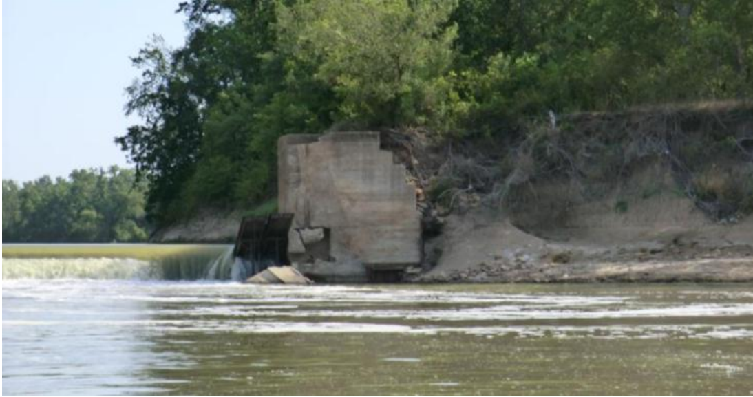
Figure 17. 080444 – Looking upstream at left bank, from below USACE Lock 3; July 2011, prior to flanking.
