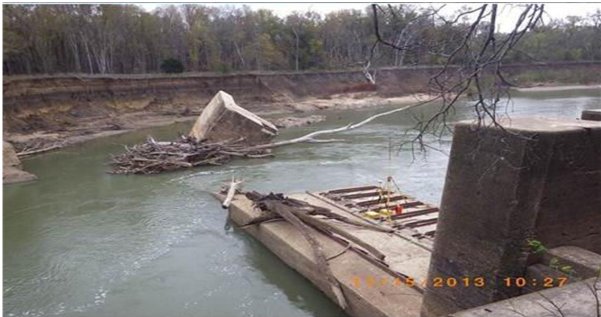
Figure 23. Photograph showing the river flanking the historic lock structure. Downstream is towards the right.
