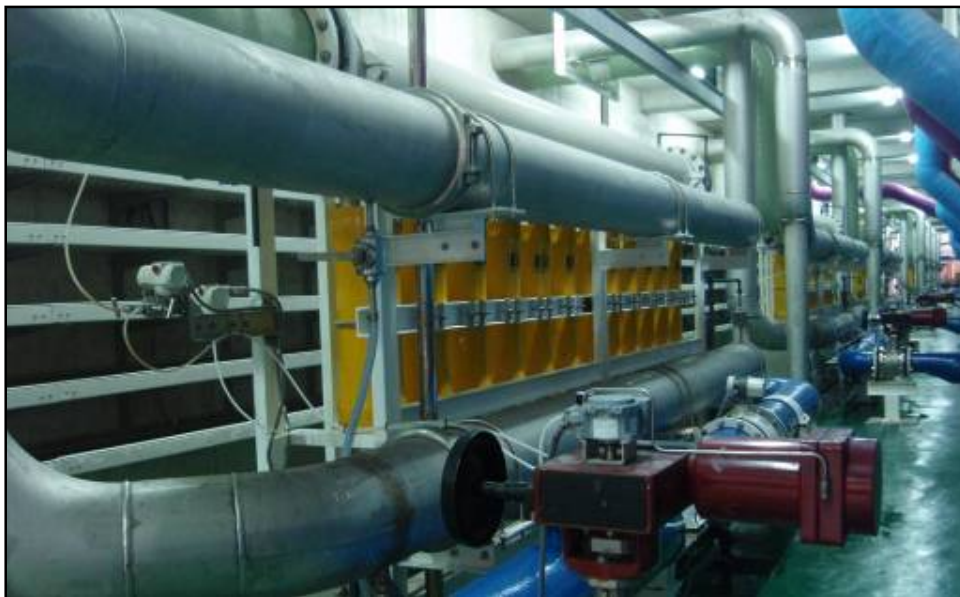
Figure 2 – PX Energy Recovery Device Array
